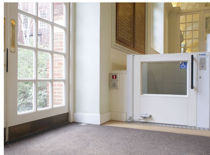
Lift no.20 – ground floor
